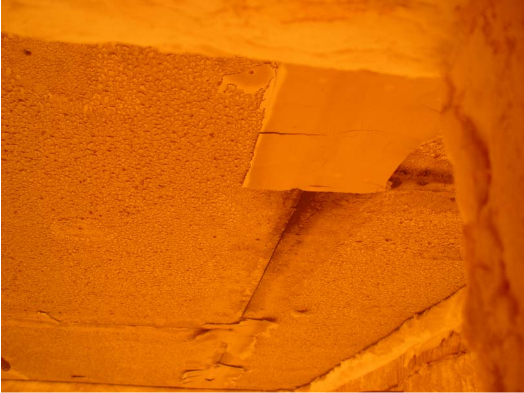
15 minutes- tape falling from E-W joint at N end of furnace
