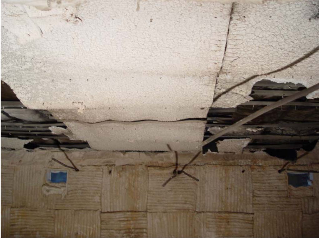
Post test: center section of ceiling
